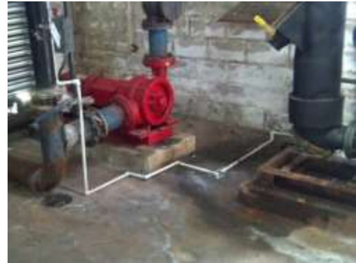
Moisture in Concrete Slab
